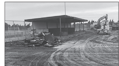
Maintenance /Transportation Garage – Removal of the existing asphalt at the Maintenance/Transportation Garage.
